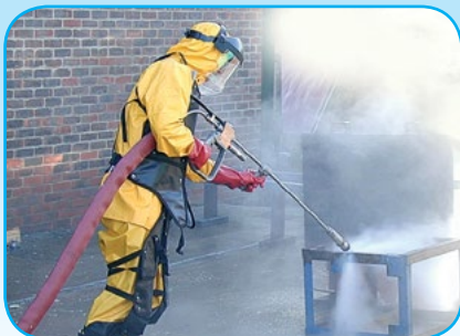
De-scaling - 28lpm / 1400 bar
