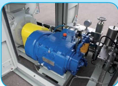
Pump fitted with switches & connected to a high pressure manifold with a pulsation damper & control valves
