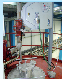
Hosereel to lower/raise tank nozzle
