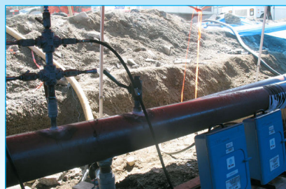
Pipeline monitoring station
