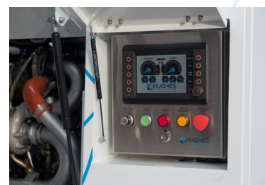
Comprehensive but simple control panel
